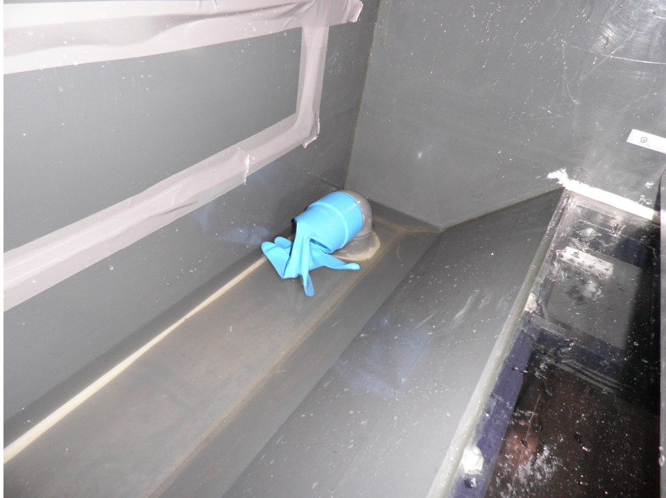
Pic. 14 Tubes blocked.
