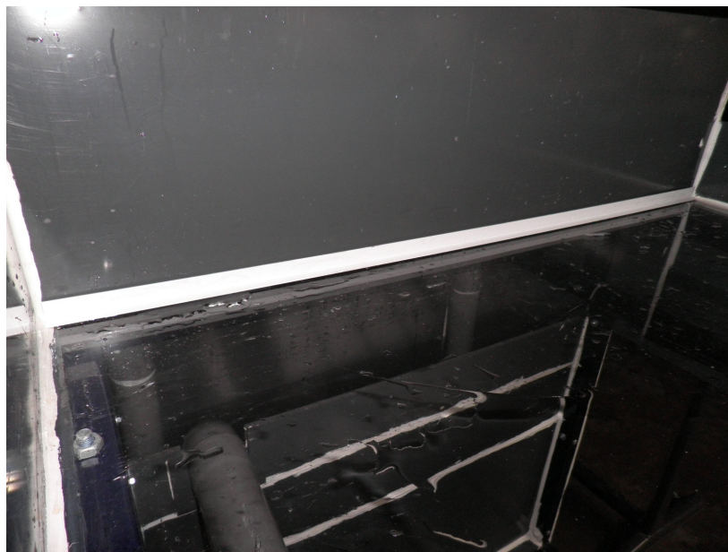
Pic. 12 Entrance blocked.
