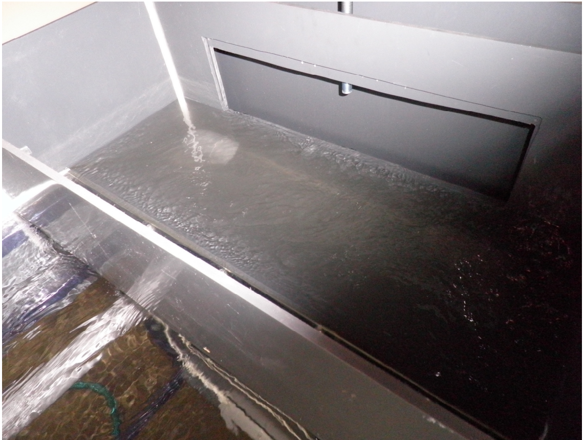
Pic. 6 The opening is completely opened and the volume of flow is still high and turbulent.
