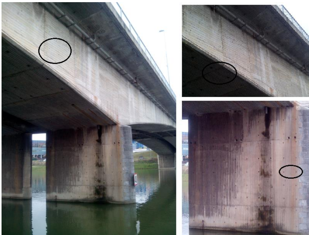
Figure 3: holes in bridges
