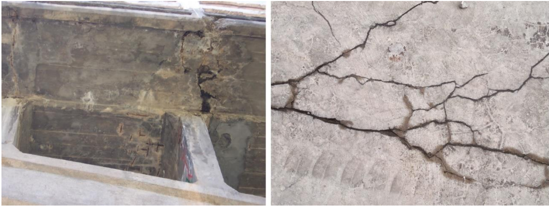
Figure 2: Cracking in surfaces made of concrete
