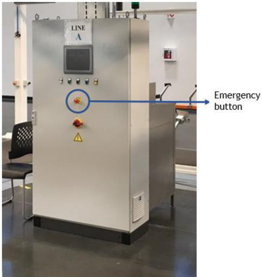
Figure 5.4: Emergency button's location
