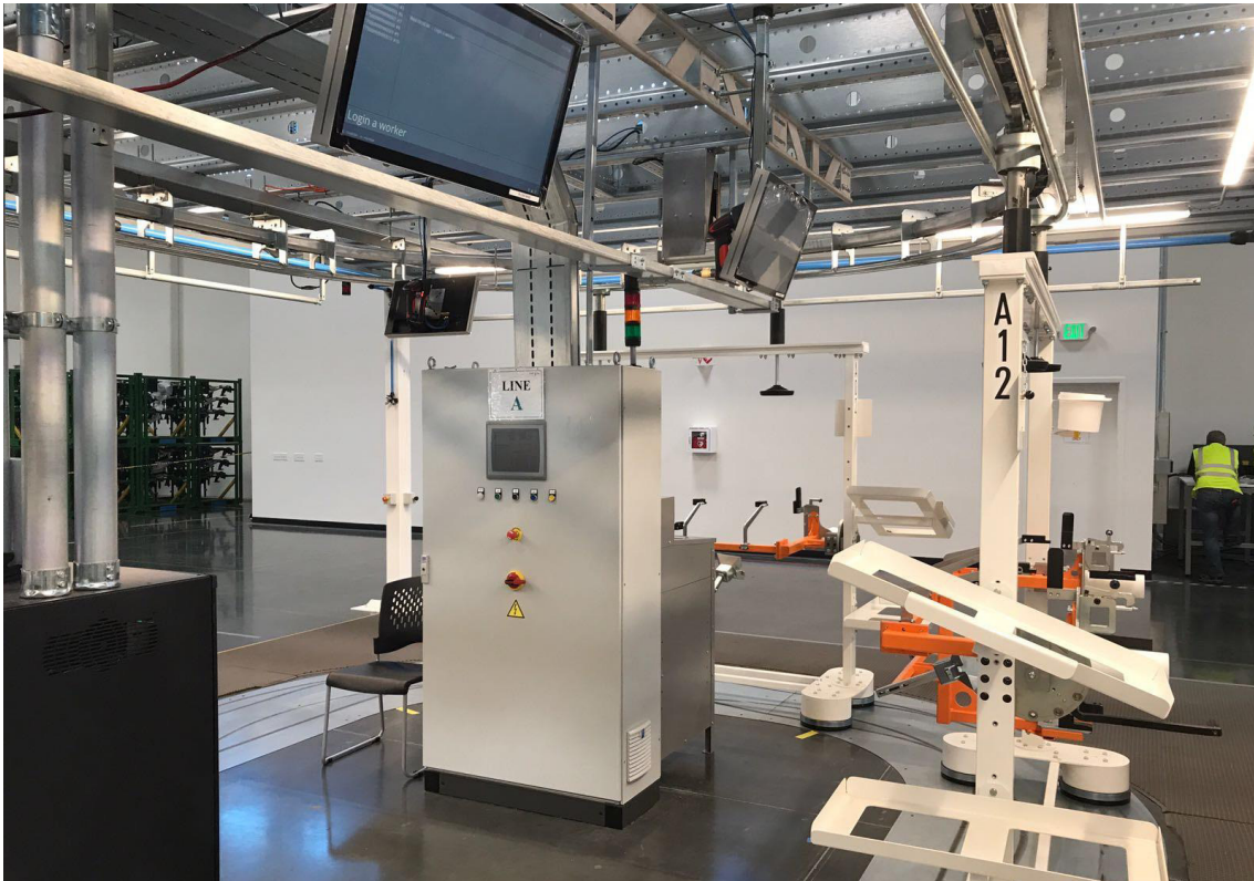
Figure 4.30: Newark's Electrical cabinet
