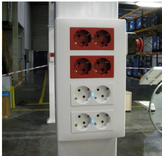
Figure 4.32: Example of red and White sockets (Germany)
