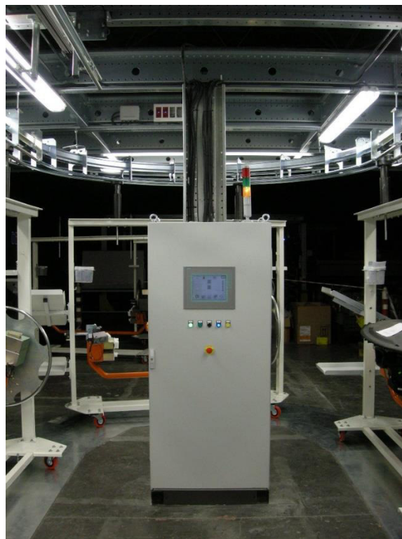
Figure 2.5: Example of an electrical cabinet with the HMI and the push buttons
