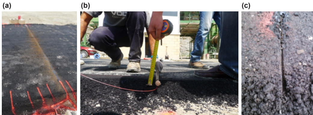
Figure 6.19. Pictures of the asphalt platform including optical fibers just before the sensitivity test.
