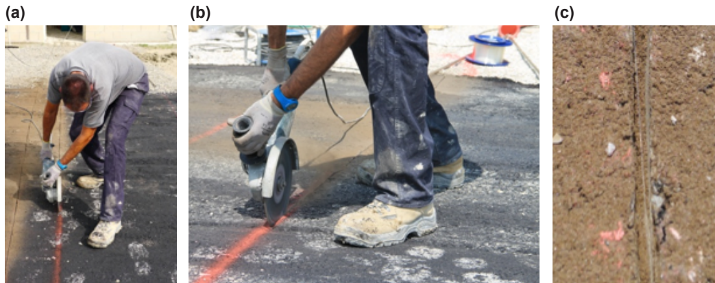
Figure 6.17. Pictures of the fibers installation in asphalt. (a) and (b) are pictures of the groove opening and (c) is how the fiber is placed in the trench before protecting it.
