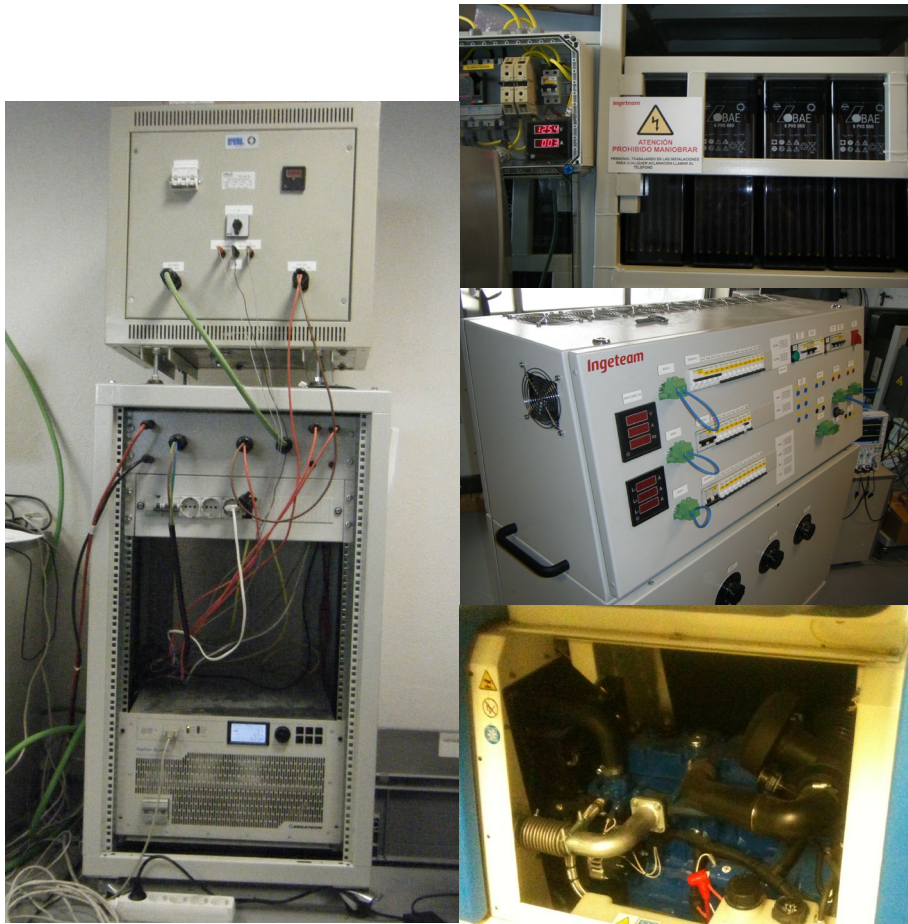
Fig. 14. PV emulator, battery inverter, PV inverter, battery bank and load bank used for the experimental setup.
