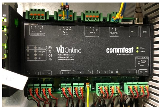
Fig. 41: vbOnline system installed
