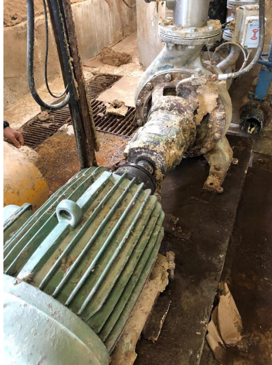
Fig. 64: Refine pump and its motor
