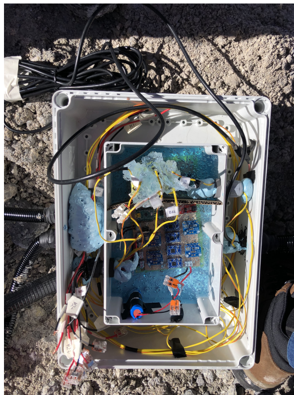
Figure 8. Detail of the protection boxes to avoid corrosion in the PCB.
