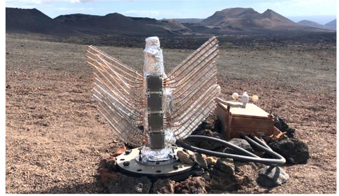
Fig. 14. Geothermal thermoelectric generator for high temperature geothermal anomalies installed in Islole Hilario (Timanfaya National Park, Lanzarote).
