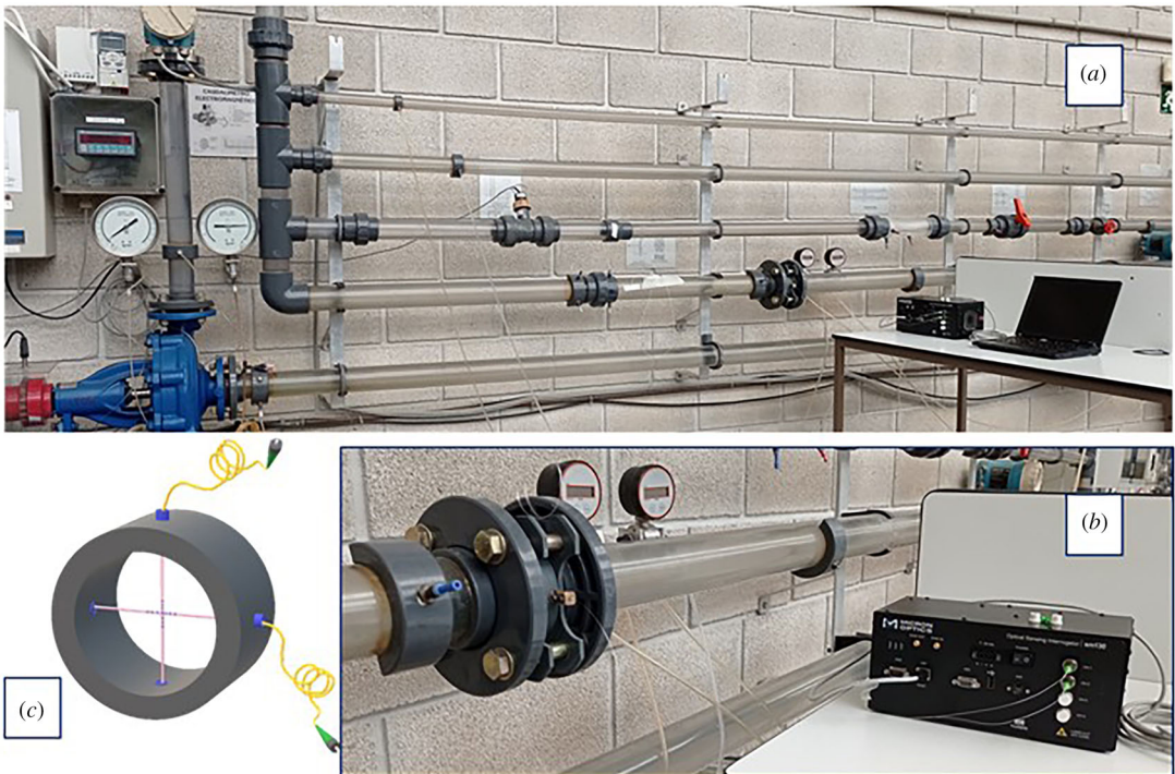
Figure 5. (a) Pipe panel on which the experiment has been carried out; (b) mechanism for the installation of the sensors in the pipe; (c) Detail of the placement of the sensors in the support designed for the experiment.
