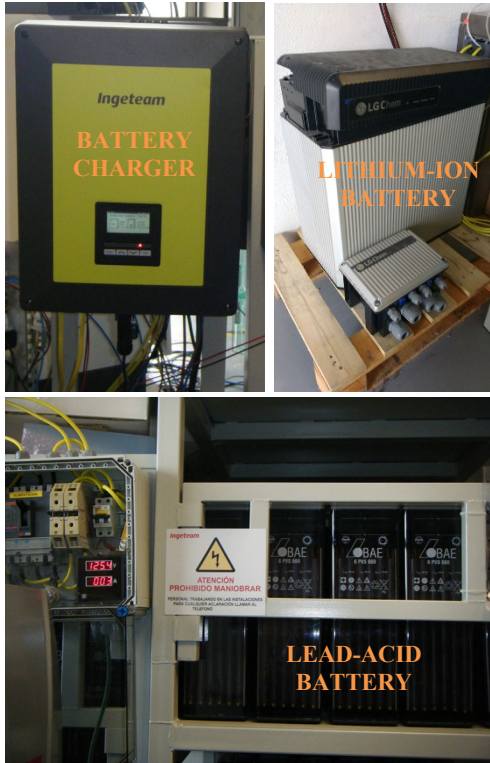
Fig. 14. Battery charger, lithium-ion battery and lead-acid battery used for the experimental setup.
