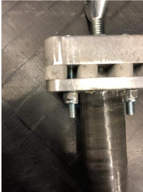
80 [Problematic built pushrod]
