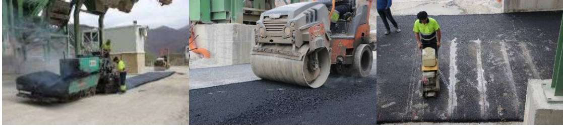
Fig. 2. Pictures of the asphalt paving procedure and trenching for the fibers installation.
