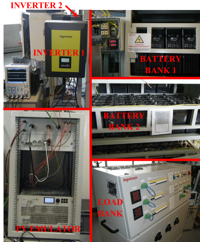
Fig. 13. PV emulator, battery banks and load bank used for the experimental setup
