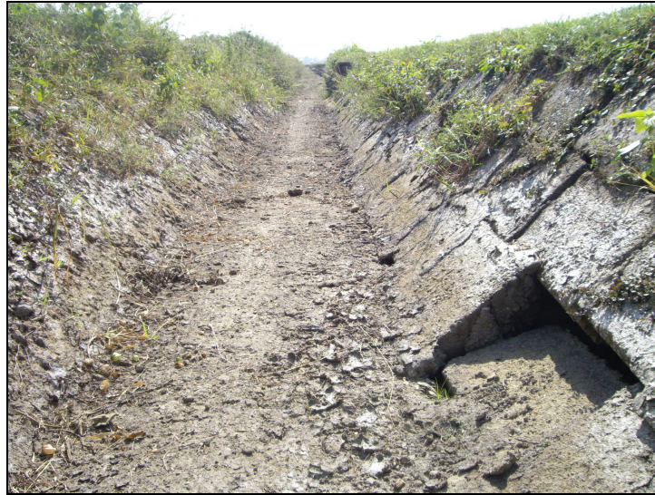
Image 6: Brick masonry deterioration in the mid part of Main Canal.
