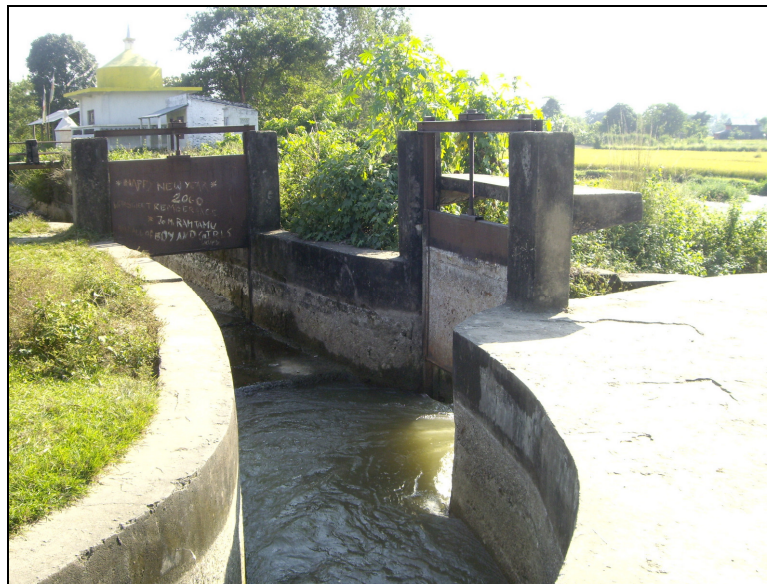
Image 2 Escape structure (right) and Head Regulator (left)
