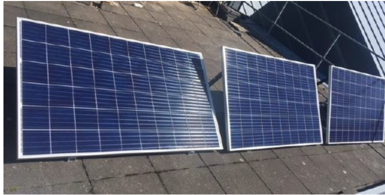
Figure 3.1.3. Tilt angle adjustment of the PV panels (7)
