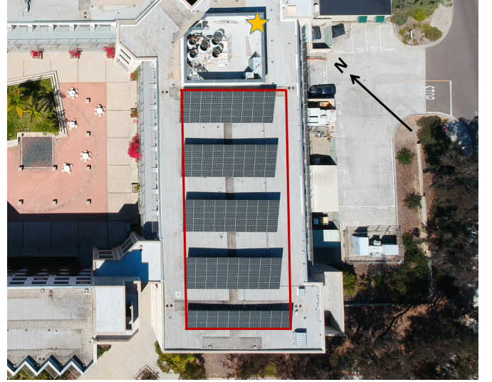
Fig. 2. Aerial view of the PV system installed on EBU2 at UCSD and the PV production field (red) considered in this paper. The yellow star indicates the CSS located 10 meters north of the upper corner of the PV system. ©Drone Photo
