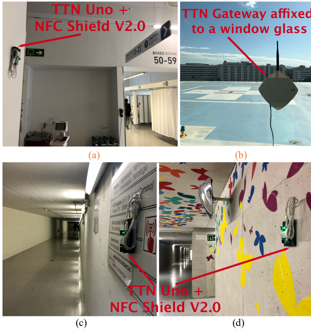
Fig. 8. LoRaWAN system deployment. Devices location at the: (a) RX building; (b) ER building; (c) Tunnel 2; (d) Tunnel 1.
