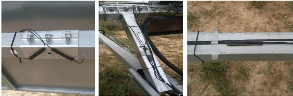
Fig. 3. Picture of three installed sensors: a) T1 b) S1 c) S2
