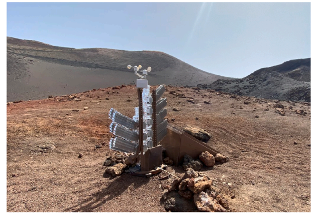
Fig. 2. Geothermal thermoelectric generator for medium temperature geothermal anomalies installed in Casa de los Camelleros , Timanfaya National Park [22].
