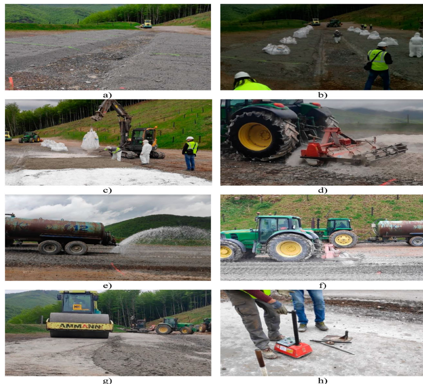
Figure 5. Field trial construction. (a) gypseous soil layer, (b) binders in big-bags, (c) binders distribution, (d) dry soil-binder mixing, (e) layer watering, (f) wet soil-binder mixing, (g) layer compaction and (h) layer density and moisture control.
